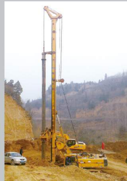
陇海路高架延伸荥阳段XR360施工快速高效 XR360 was working in Longhai railway with high working efficiency
