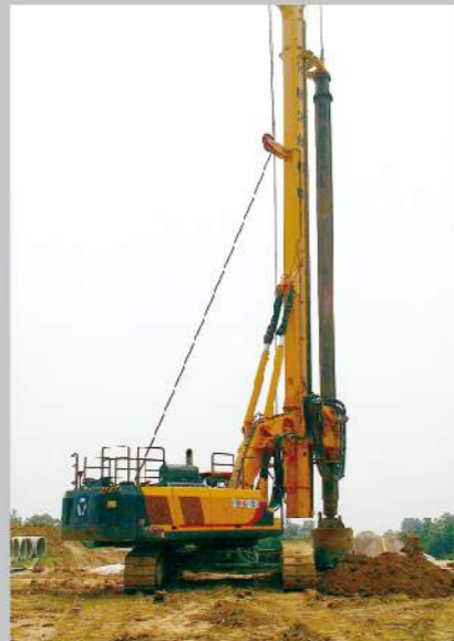
陇海路高架延伸荥阳段，施工快速高效 XCMG rotary drilling rigs were working in express way with high efficiency
