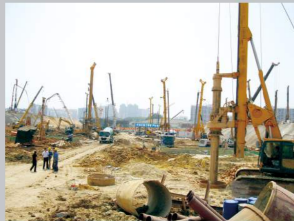
徐工旋挖钻机在南宁火车站施工 XCMG rotary drilling rigs are working in Nanning Train Station
